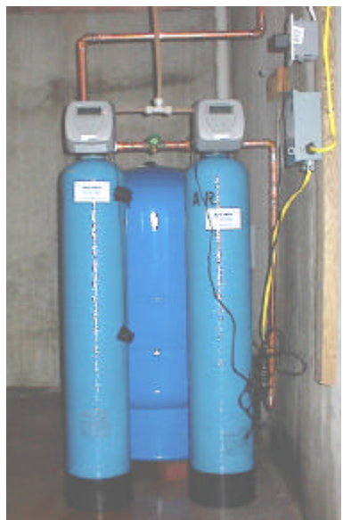
Use of AD33 media in typical point-of-entry system installation. Picture courtesy of Aquamech, Inc.
